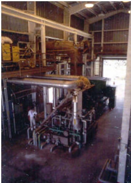
Figure 3. The HGP-A power plant showing the generator and turbine set inside the building (Lund, 1985).
